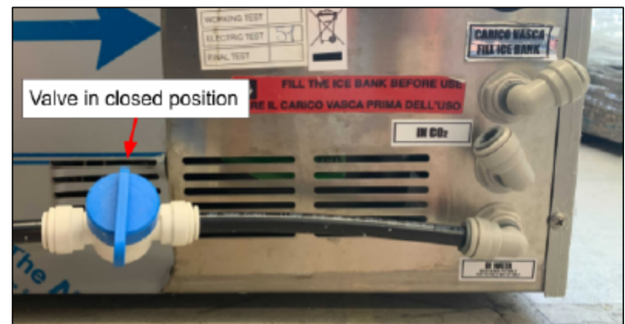
Fill Valve located at rear of Chiller
